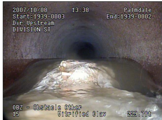
Photo: 2463, Tape/Media No.: A315-011, 00:09:35 229.7FT, Obstacle Other, from 3 to 9 o'clock, 40 %, within 8 inch: NO, Remarks: DEBRIS
